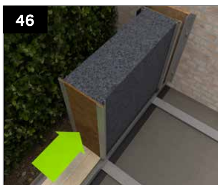
Attach half clips and position the first walling panel in place following the standard process as shown from step 21 and 22, securing the host wall tray and base trays together.
