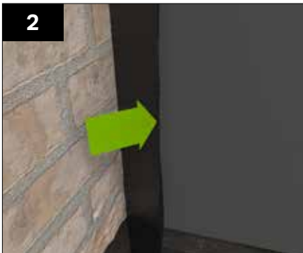
2 At the host wall fold the vertical DPC over the top of the membrane prior to battening out.
