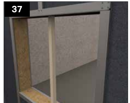
Leave the prop in place, this can be removed later once the clips are secure into the beam or tray above (roof dependant).
