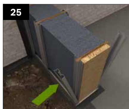
Fit the walling panel and aperture panel together using the steel full clips, using the same method as previously used for attaching walling panels together.
