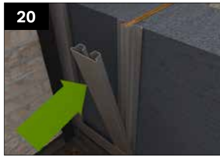
Secure the two panels together using the steel full clips. This can be done by knocking the clips onto the panel, it is helpful for a second person to brace the opposing side whilst this is being done.
