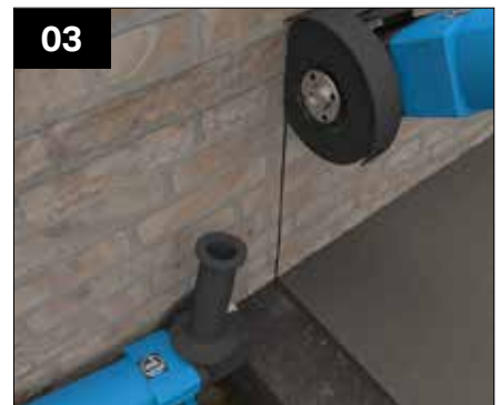
03 Install a vertical DPC suitable for the local environmental conditions to create a continuous cavity, 25mm cut out for the DPC is required.
