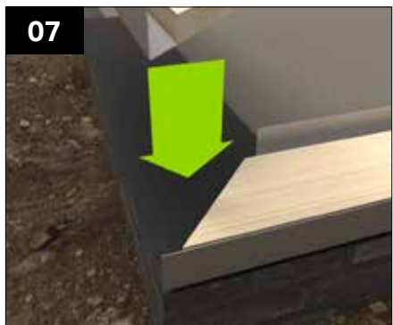
07 Referring to the location plan, loosely position the base trays on top of the DPC. Where walls are to be positioned, the DPC should run past the base trays, by minimum of 50mm, allowing for it to be lapped up the aperture face of walling.
